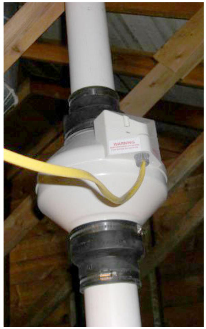
Blower fan in attic space to vent air in a radon mitigation system.
